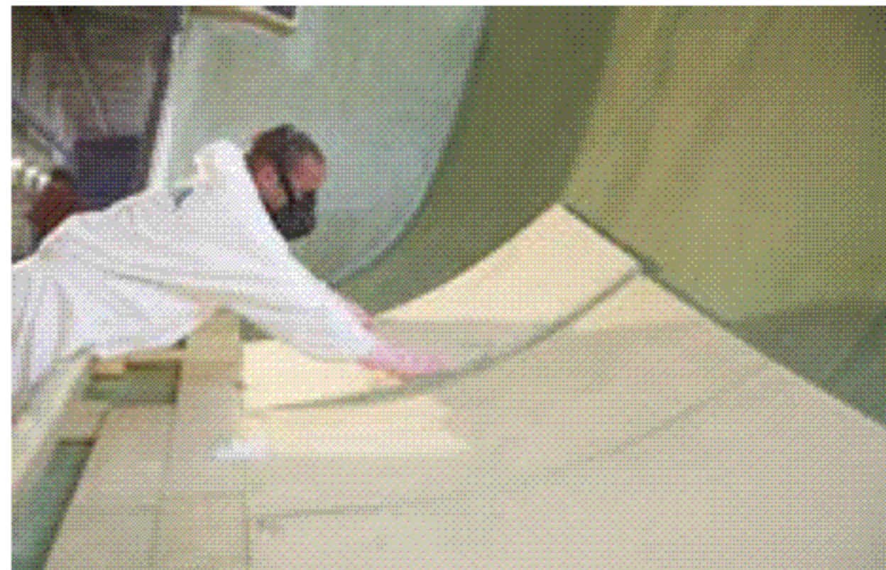
▲ The core material is added on top of the outer laminate layers of glass
