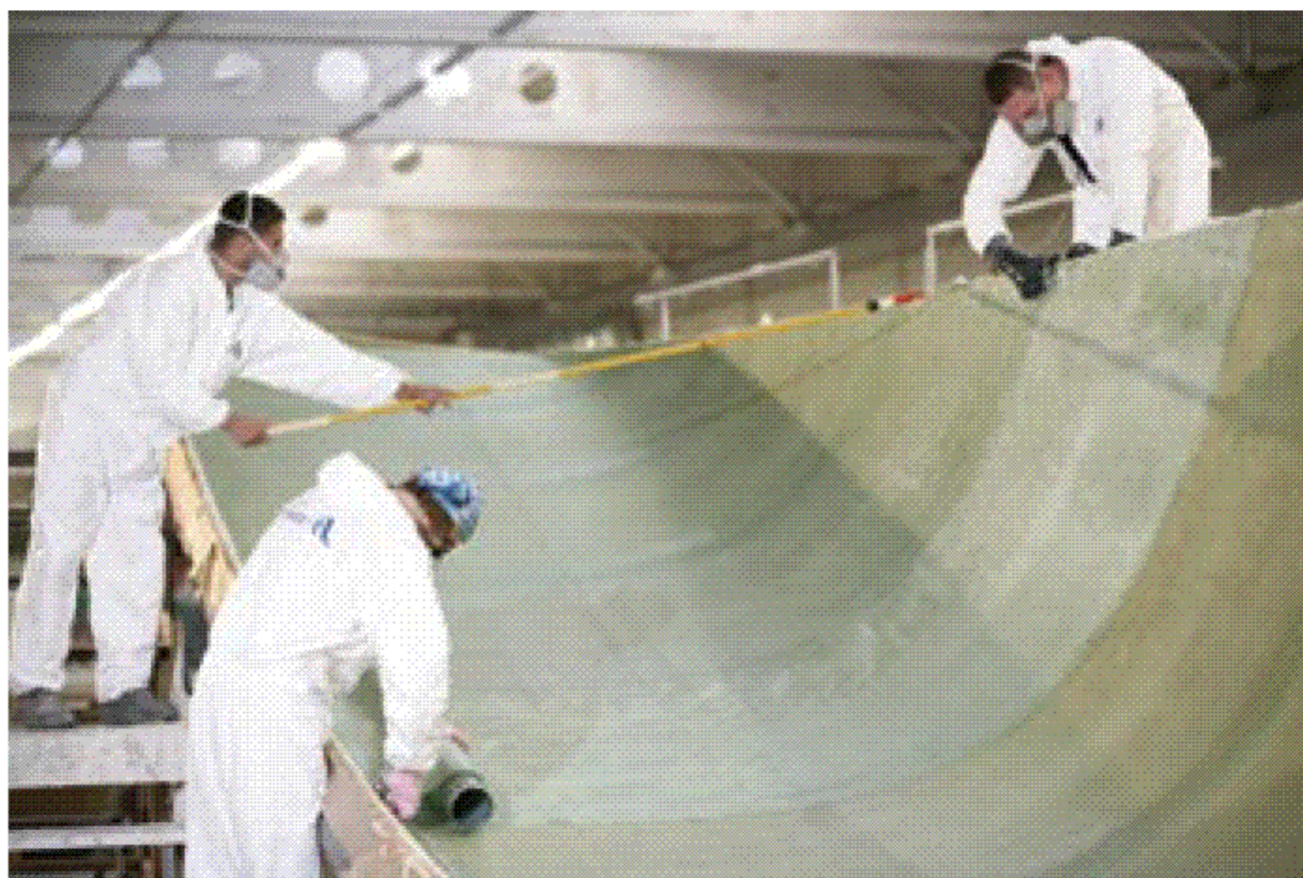
▲ The inner wetted-out glass laminates are added over the core and then consolidated with a plastic vacuum bag
